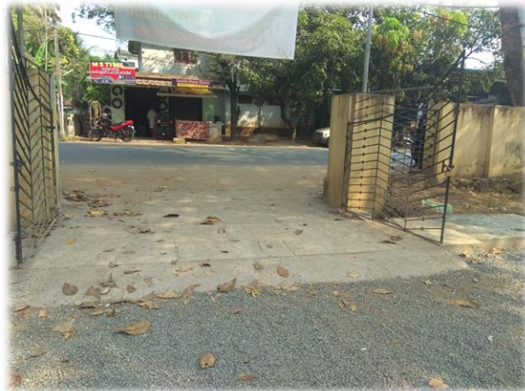
After: Constructed compound wall and repaired gates at both school entrances Government Higher Secondary School, Kuttamassery
