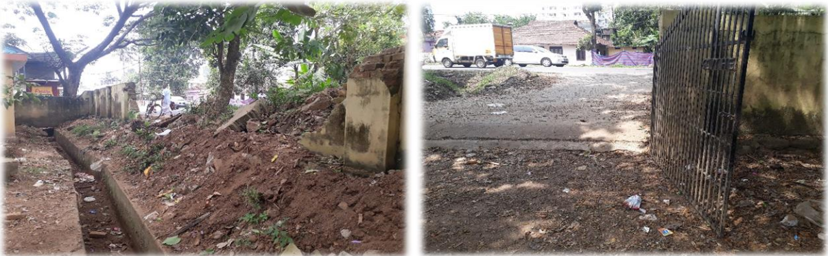
Before: The floods completely damaged the front compound wall of the school and created uneven slops in entrance slabs and gaps in gates Government Higher Secondary School, Kuttamassery
